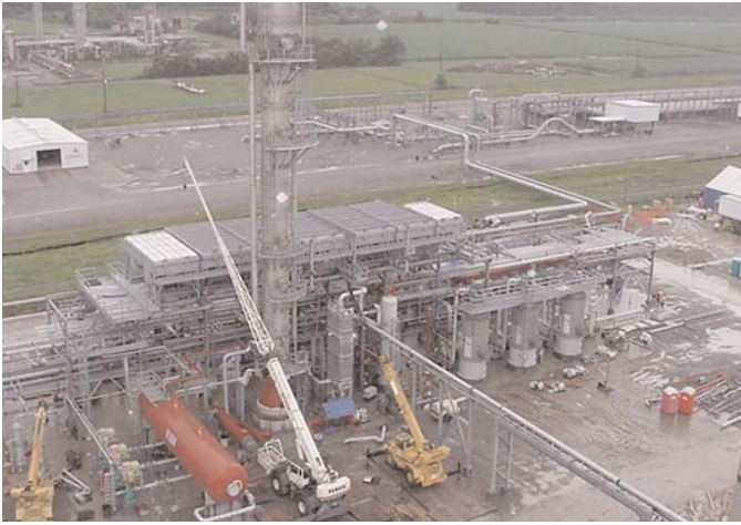
The Neptune II unit, currently under construction, will double the plant's capacity. Photo courtesy of Enterprise Products Operating LP.
